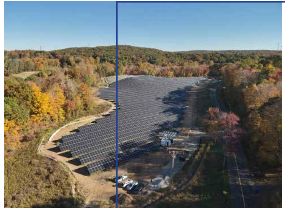
Johnson Lane Solar Farm
