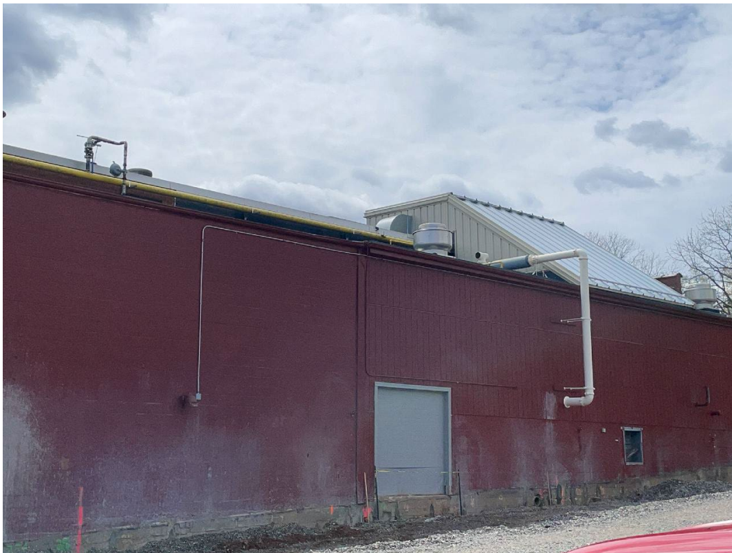
SSDS components on the side of the main DMC building
