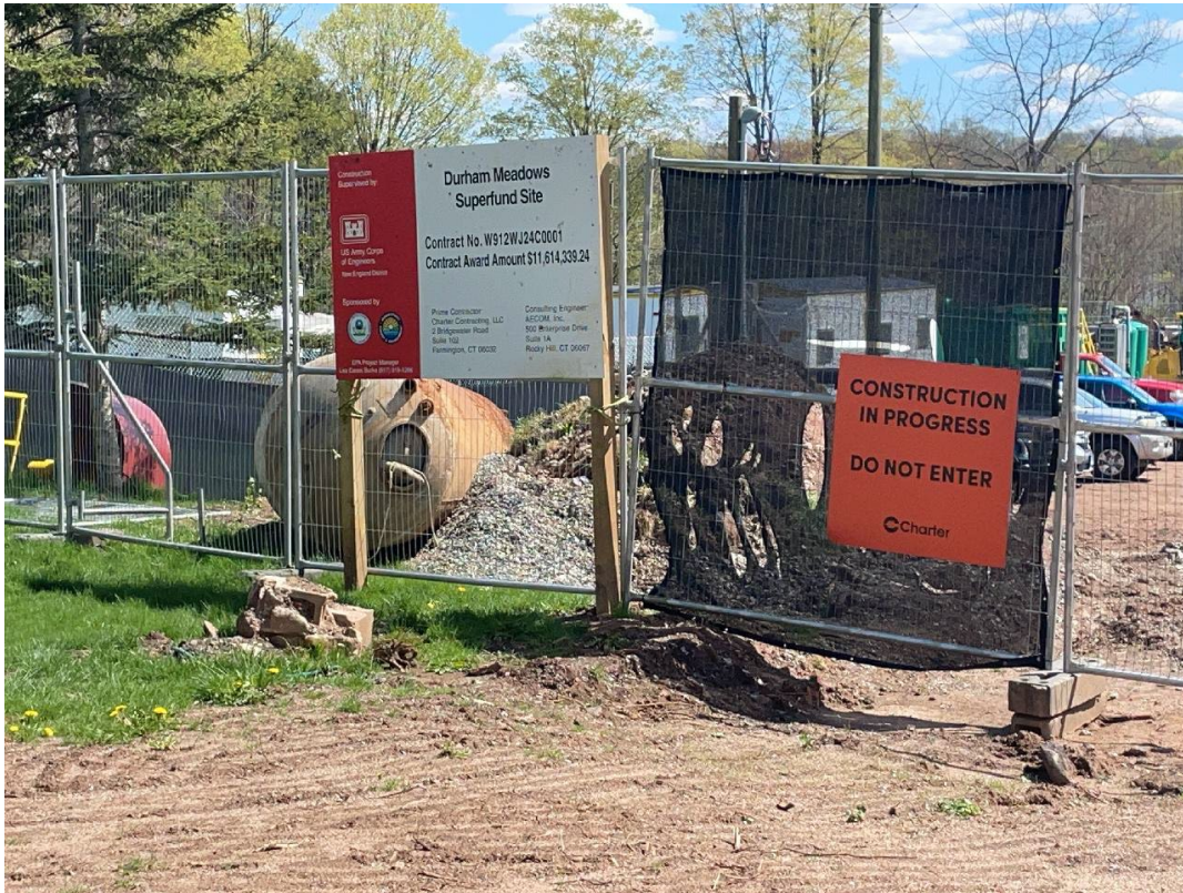
Sign and fence at the entrance to the DMC Study Area
