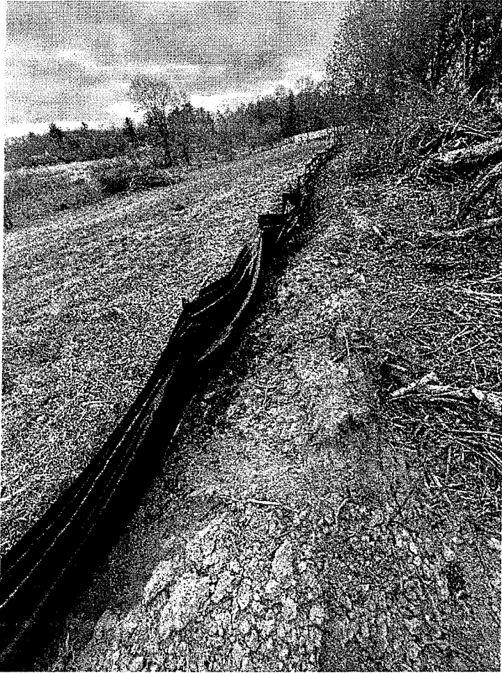
70 Newcomb Rd. Work started. Silt fence not backfilled. Owner will fix.
