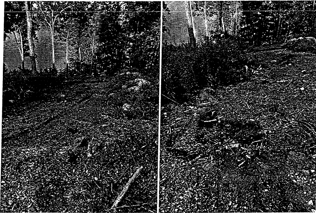
411 Milton Road, JULY Photos for reference : Some erosion/rills after rain events. Wattles installed.
