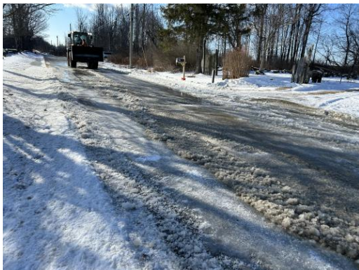
Staff removing ice across road from water pipe break
