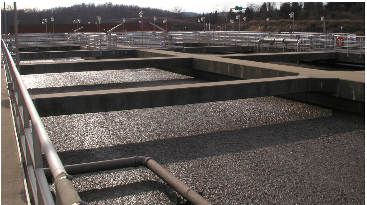
Water Pollution Control Authority
