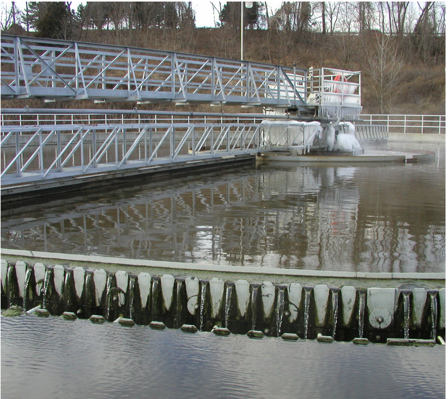
Water Pollution Control Authority
