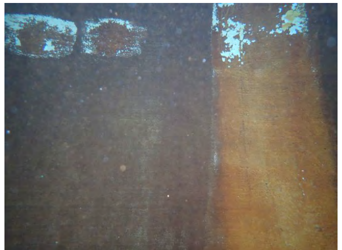
42 Interior Wall With Heavy Staining
