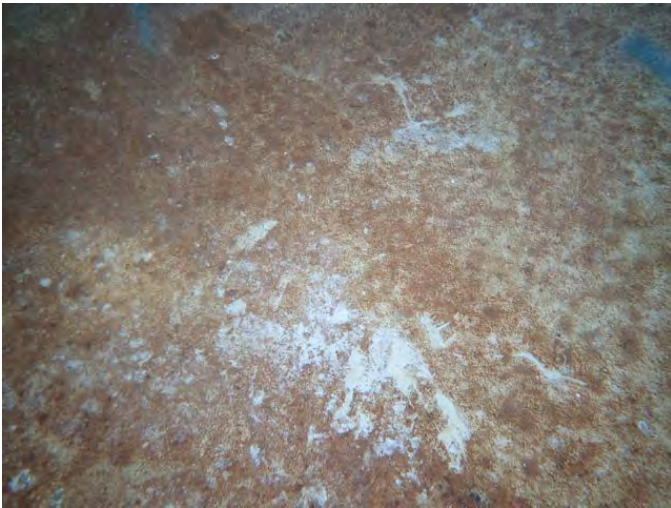
33 Floor With Heavy Staining
