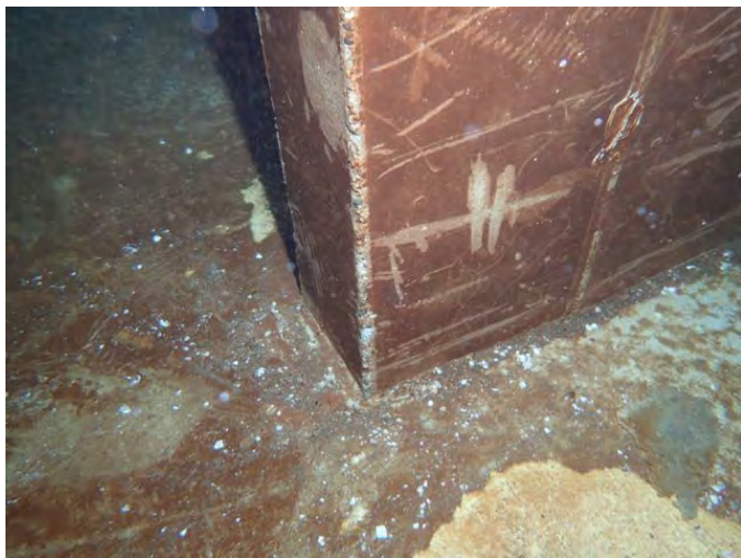
61 Baffle Wall With Heavy Staining
