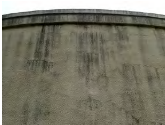
9 Exterior Wall With Coating Loss, Tight Shrinkage Cracks And Mild Mildew
