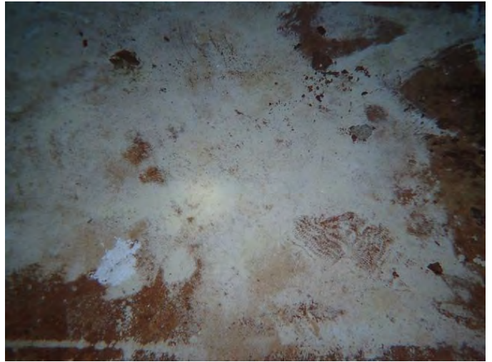
32 Floor With Heavy Staining
