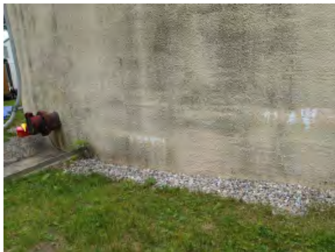
11 Northernmost Exterior Wall With Coating Loss, Tight Shrinkage Cracks, Efflorescence And Mild Mildew
