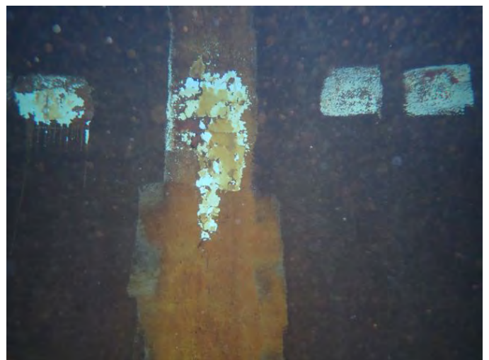
48 Interior Wall With Heavy Staining
