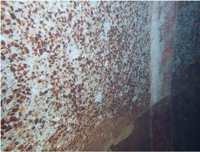
55 Interior Wall With Concrete Scour And Heavy Staining
