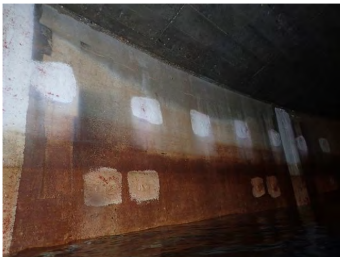
47 Interior Wall With Heavy Staining
