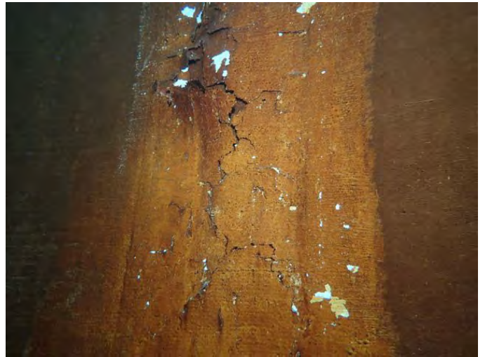
52 Interior Wall Concrete Filled Joints With Coating Loss/Cracking/Lifting, Exposed Underlying Concrete And Heavy Staining
