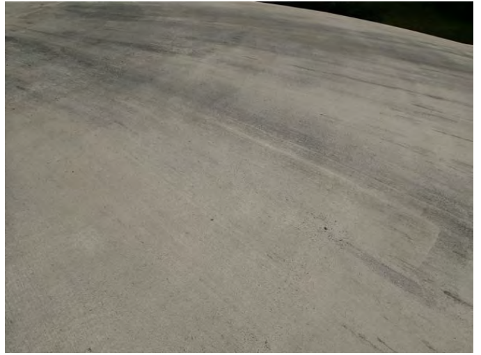
20 Roof Dome With Mild Mildew
