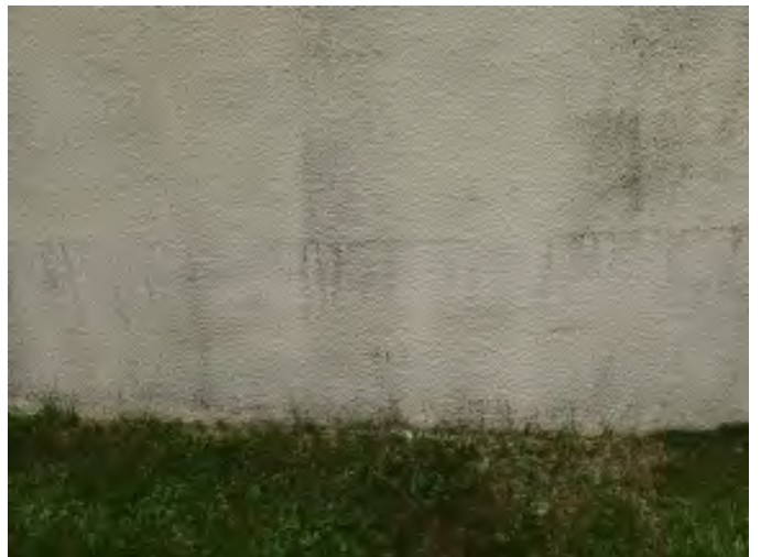
6 Exterior Wall With Coating Loss, Tight Shrinkage Cracks And Mild Mildew
