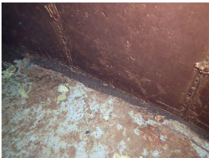
64 Baffle Wall With Heavy Staining
