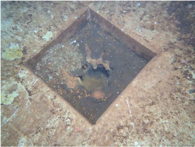
37 10" Inside Diameter Pipe - Flush Penetration Within A Deep Sump
