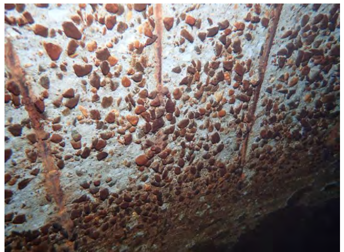
60 Easternmost Interior Wall With Concrete Scour, Exposed Reinforcement Steel, Mild Corrosion And Heavy Staining
