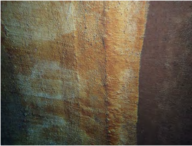
49 Interior Wall Concrete Filled Joints With Heavy Staining
