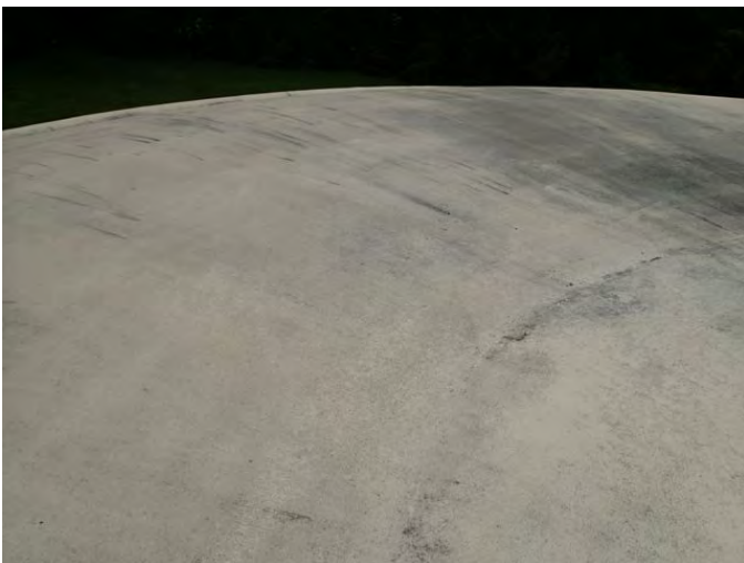
17 Roof Dome With Mild Mildew
