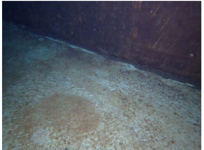
34 Floor With Heavy Staining
