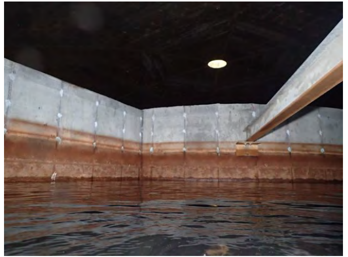
74 Aluminum Support Beams
