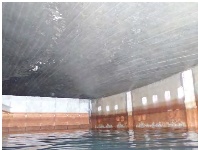
82 Overhead With Tight Cracks And Efflorescence
