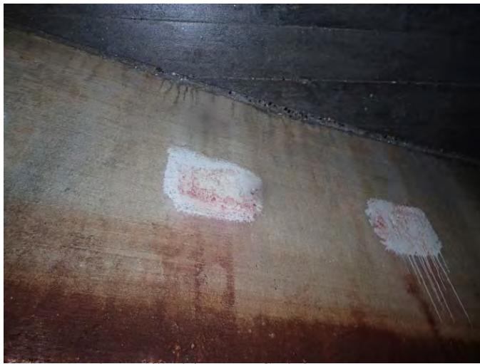
45 Interior Wall With Heavy Staining
