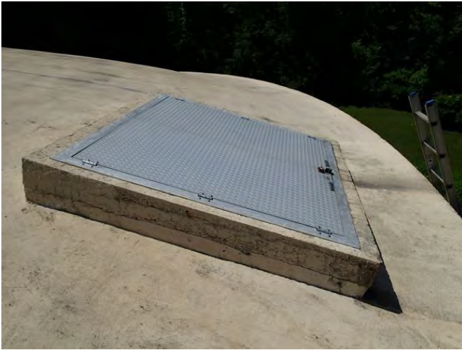
25 Closed Access Hatch
