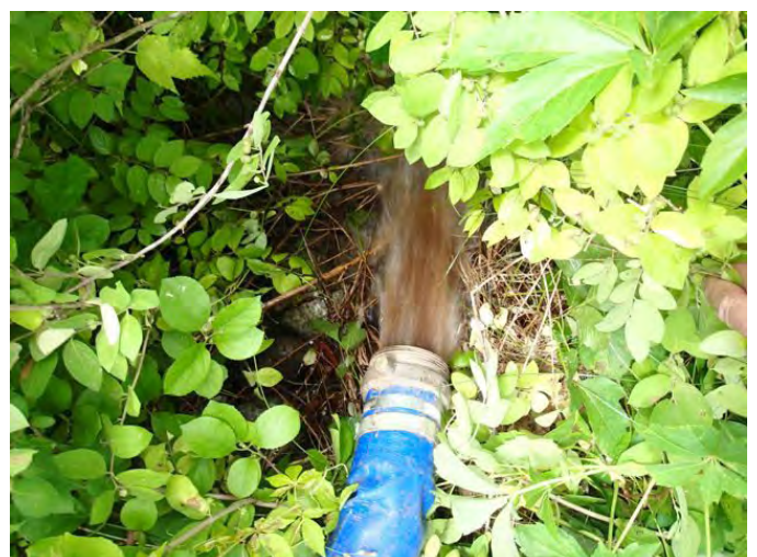
90 Discharge During Cleaning
