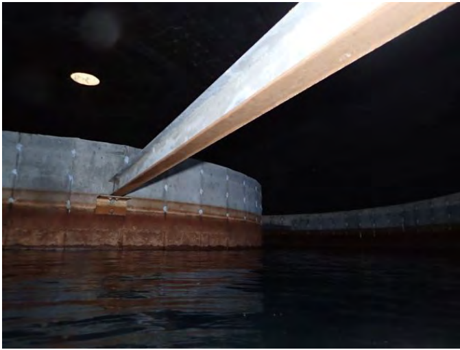
73 Aluminum Support Beams
