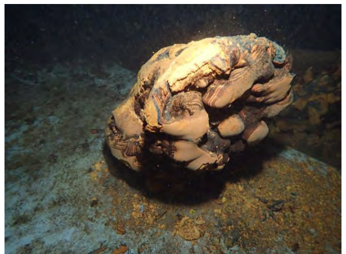
40 3" Inside Diameter Pipe Penetrating The Tank Floor With Corrosion
