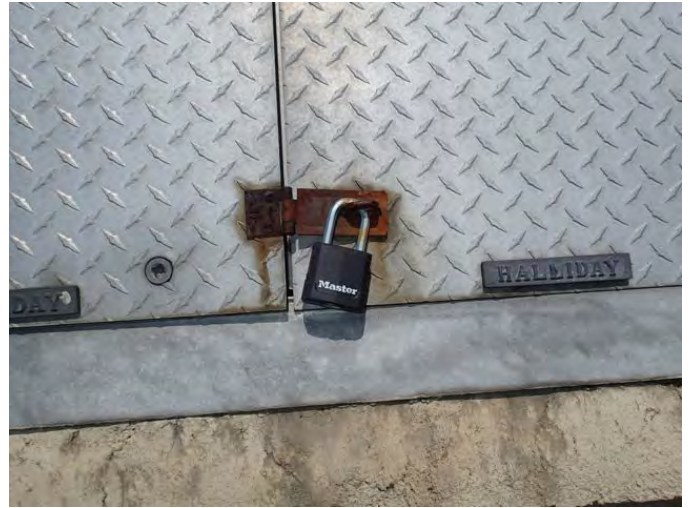
26 Secure Access Hatch
