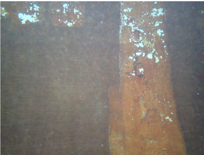
51 Interior Wall Concrete Filled Joints With Coating Loss/Cracking/Lifting, Exposed Underlying Concrete And Heavy Staining
