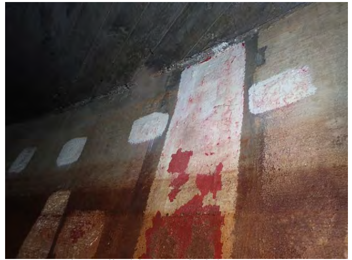
46 Interior Wall With Heavy Staining
