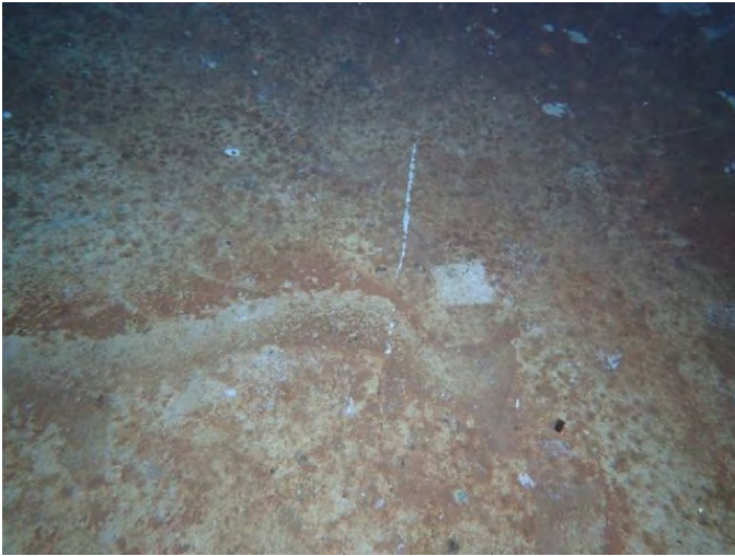
31 Floor With Heavy Staining
