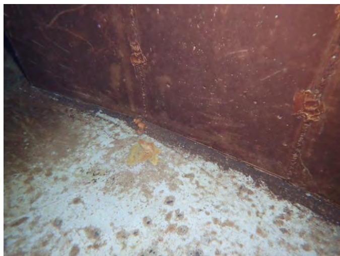
65 Baffle Wall With Heavy Staining
