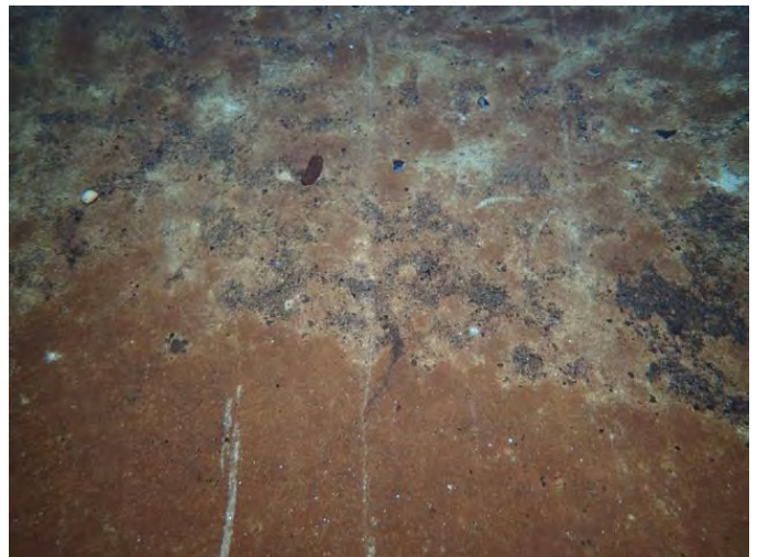
36 Floor With Heavy Staining
