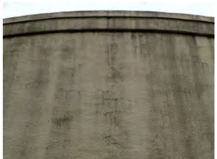
10 Exterior Wall With Coating Loss, Tight Shrinkage Cracks And Mild Mildew
