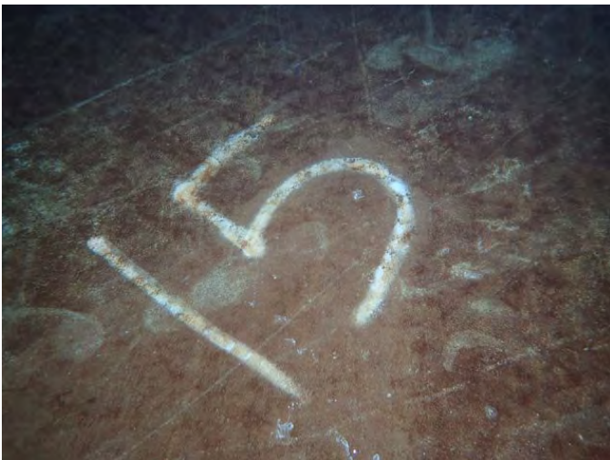
35 Floor With Heavy Staining
