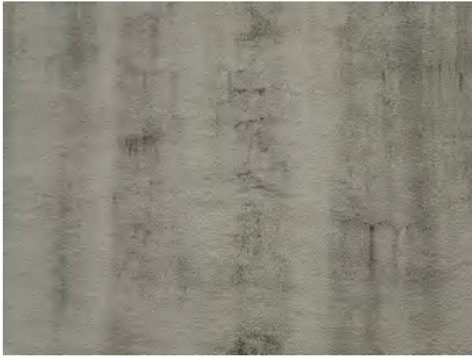
7 Exterior Wall With Coating Loss, Tight Shrinkage Cracks And Mild Mildew
