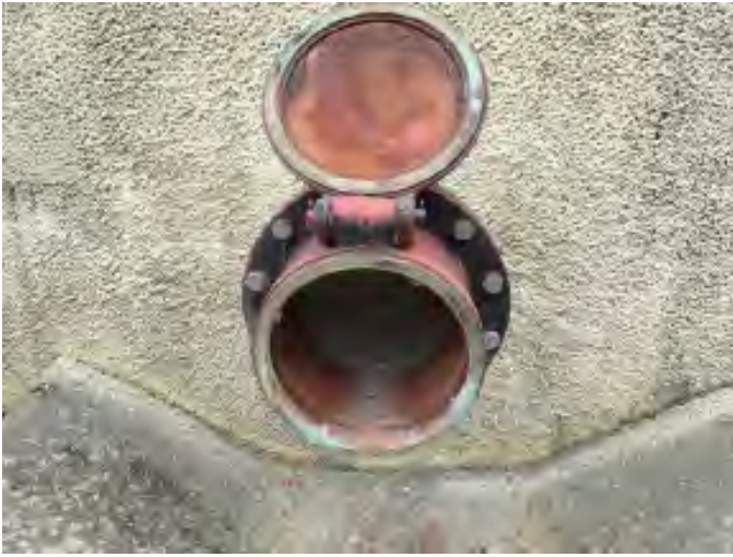
13 Overflow Pipe With A Flap-Valve
