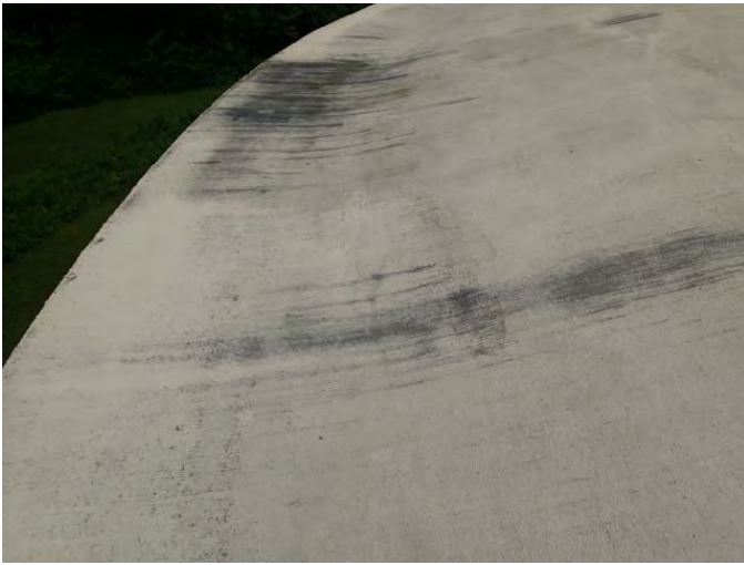
19 Roof Dome With Mild Mildew
