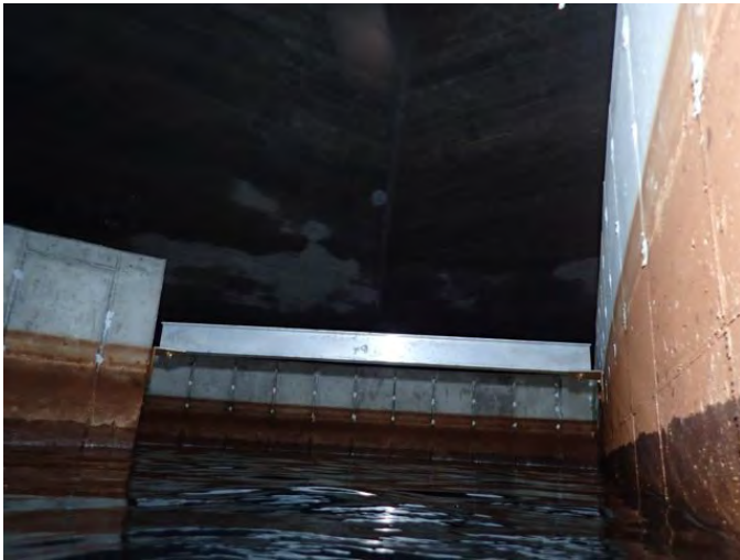
75 Aluminum Support Beams
