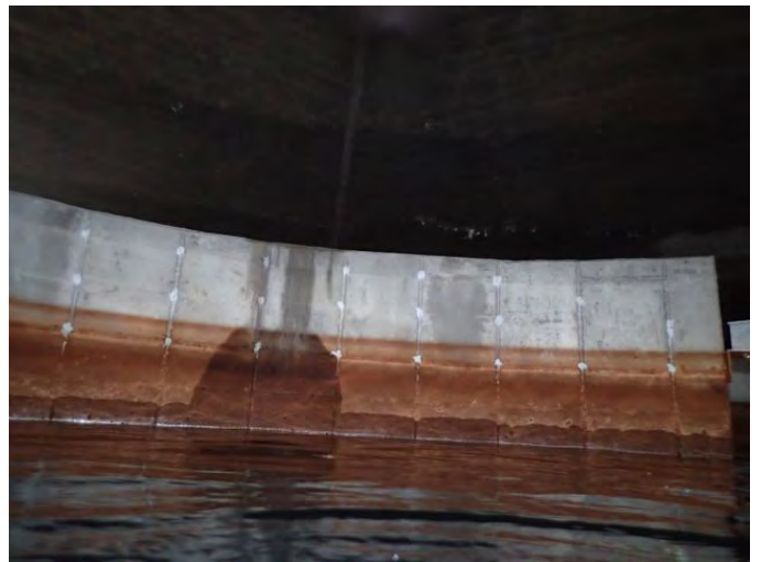
70 Baffle Wall With Heavy Staining
