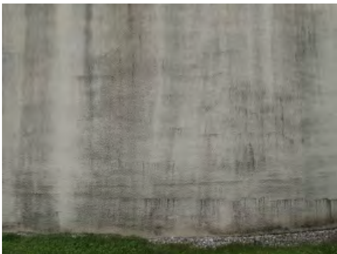
5 Exterior Wall With Coating Loss, Tight Shrinkage Cracks And Mild Mildew
