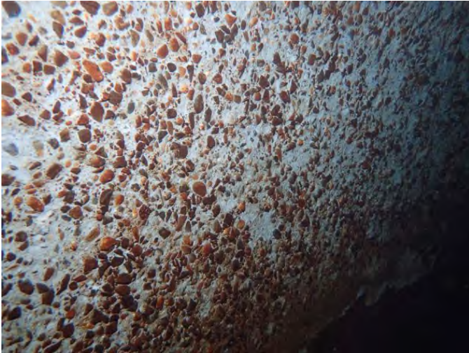
57 Interior Wall With Concrete Scour And Heavy Staining
