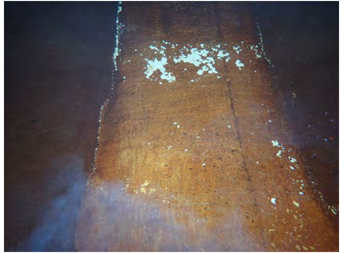
50 Interior Wall Concrete Filled Joints With Heavy Staining
