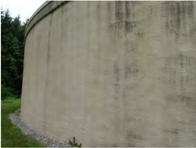
1 Exterior Wall With Coating Loss, Tight Shrinkage Cracks And Mild Mildew
