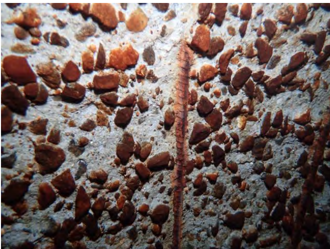
59 Easternmost Interior Wall With Concrete Scour, Exposed Reinforcement Steel, Mild Corrosion And Heavy Staining
