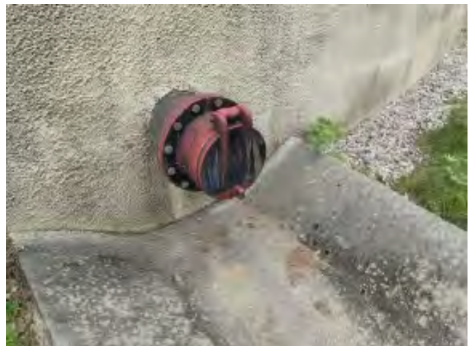
12 Overflow Pipe Terminating Above A Concrete Splash Pad
