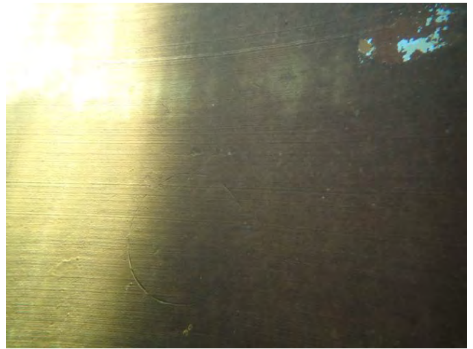
44 Interior Wall With Heavy Staining
