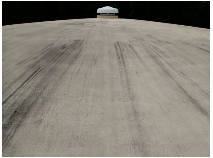
16 Roof Dome With Mild Mildew
