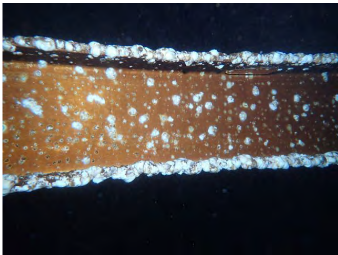
79 Aluminum Support Beams With Corrosion
