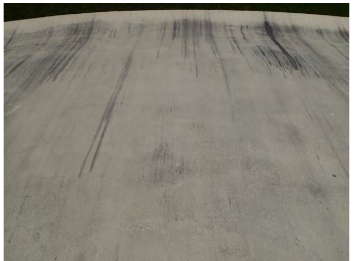
18 Roof Dome With Mild Mildew
