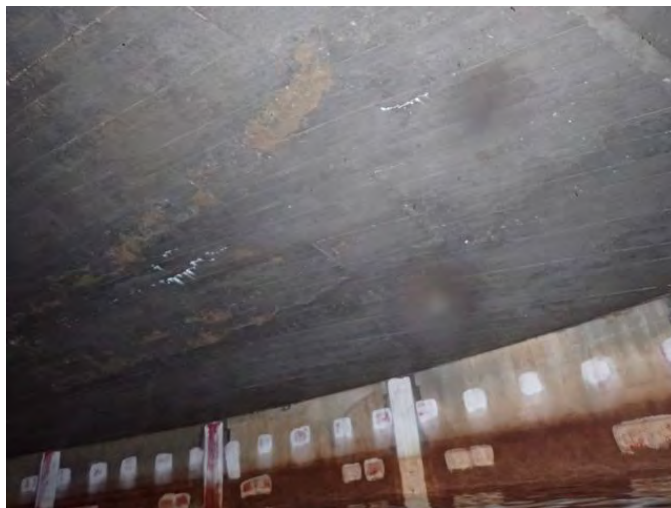
80 Overhead With Tight Cracks And Efflorescence
