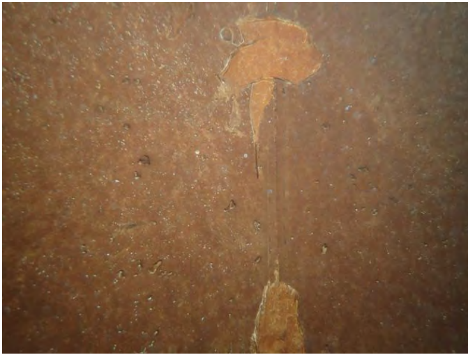
67 Baffle Wall With Heavy Staining
