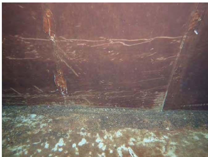
66 Baffle Wall With Heavy Staining
