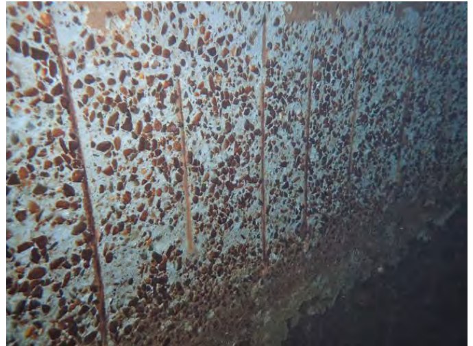
58 Easternmost Interior Wall With Concrete Scour, Exposed Reinforcement Steel, Mild Corrosion And Heavy Staining
