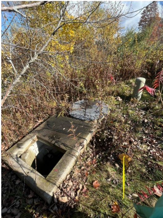
Photo 5: E1 Transformer Vault, E-Vault, Comms Equipment
