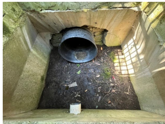
Photo 2: CB 12 parge coat missing
