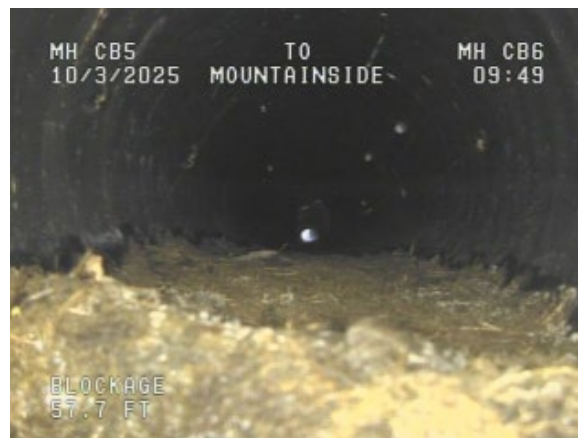
Photo 7: Blockage between CB5 and CB6
