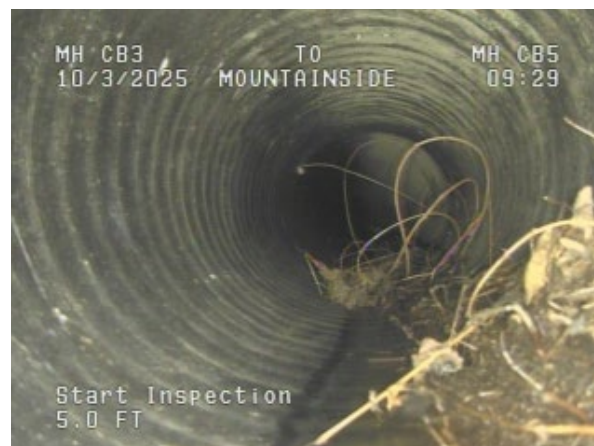
Photo 8: Root growth from CB3 into drain line
