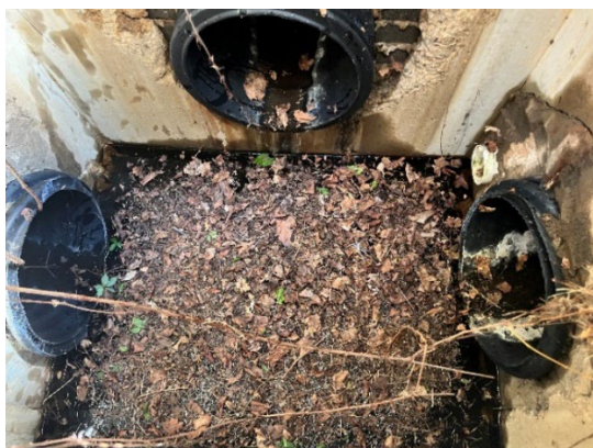
Photo 1: CB 3 parge coat issues and cracking
