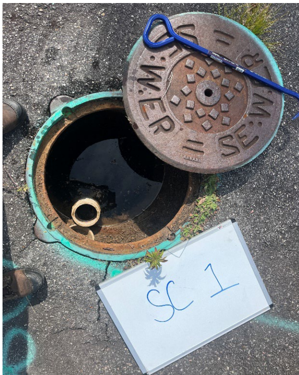
Photo 3: General water level in sewer manholes
